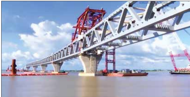
Dream of the nation the Padma multipurpose Bridge is being constructed with Railway track.
